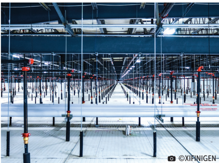
New mechanicals above ceiling in interstitial space.
